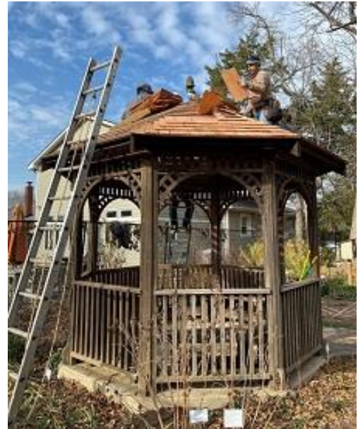
Workers from Kirby Kerns replace the Glencarlyn garden gazebo roof. (Photo/Elaine Mills)
